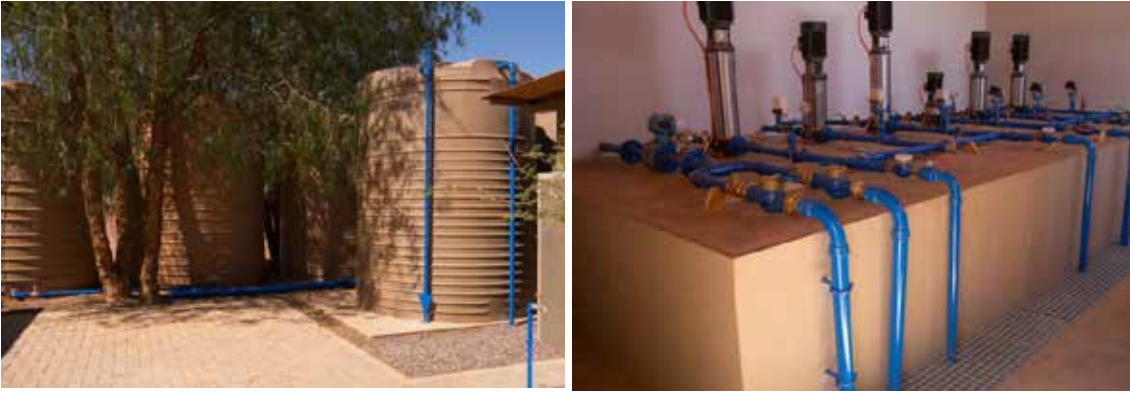
Water tanks and pumps at Wolwedans (Photos by Judith Schulze)
